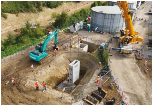
1.7M invested at the Gondardennes site to recover rainwater over 11 hectares.
