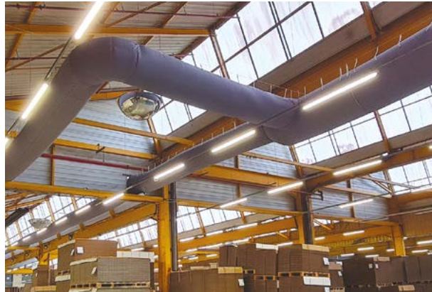
New workshop heating system.
